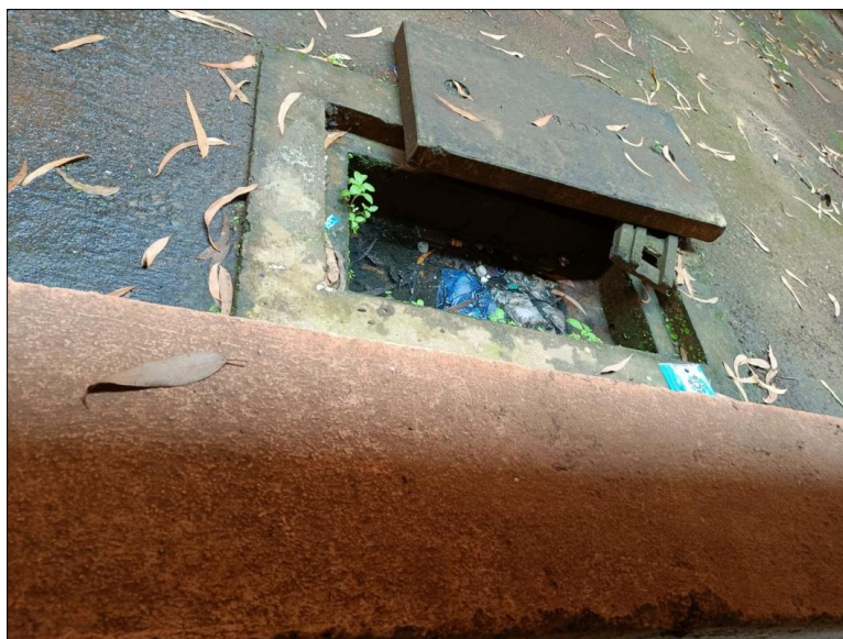
Figure 1 Common drainage site of sewage collection at District hospital Ratnagiri
